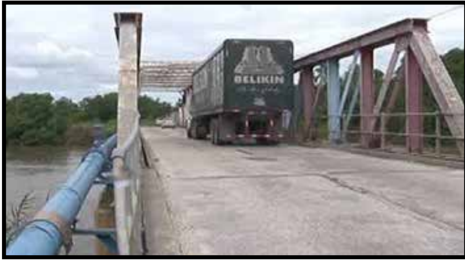
No vehicle above 22,000 lbs allowed on the bridge
